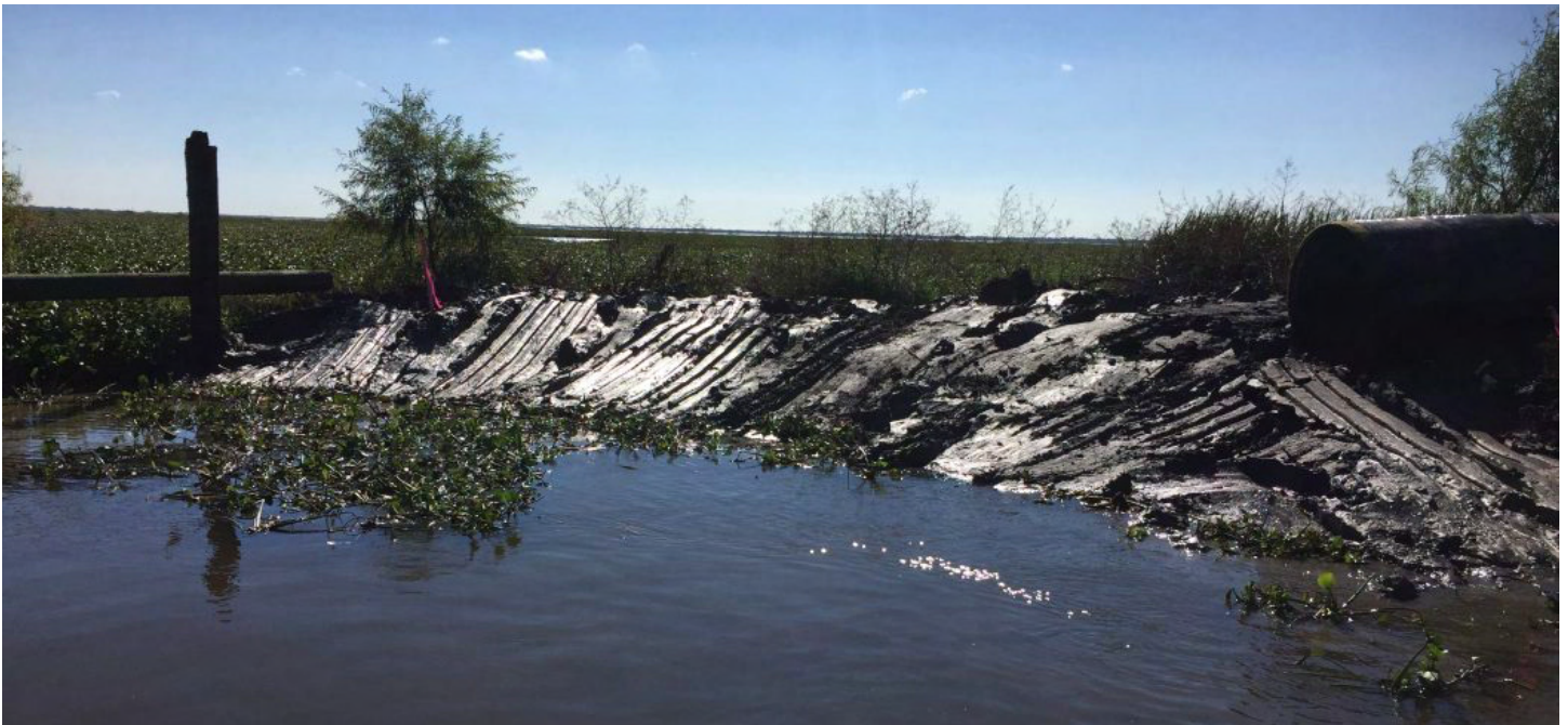
Newly created berm, ready for the installation of Vegetated EcoShield™. Courtesy America's WETLAND Foundation.
