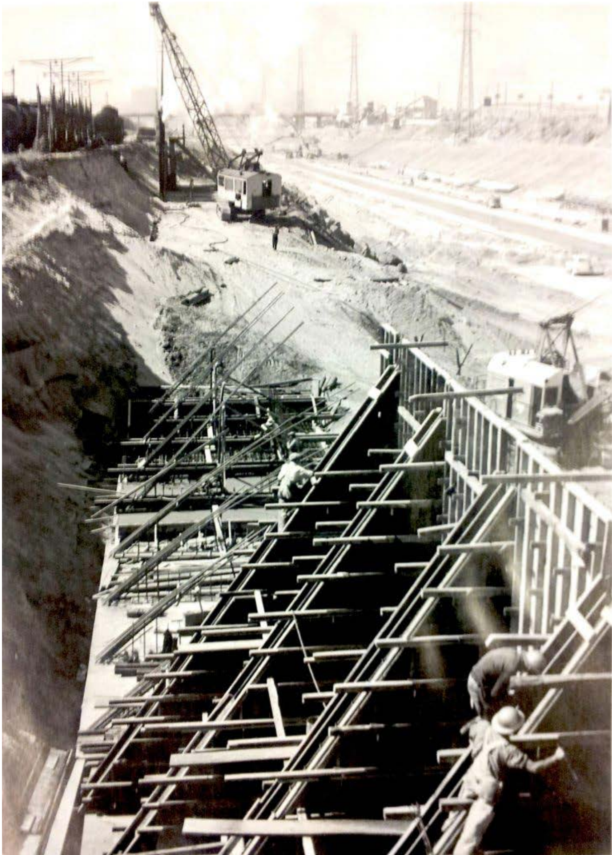
Upstream view of the Los Angeles River channel above Butte Street Bridge during construction. Image via U.S. Army Corps of Engineers Los Angeles District .
