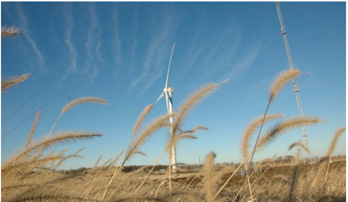
The Eolos Wind Energy Field Station consists of a fully instrumented 2.5 MW Clipper Liberty wind turbine and 400-ft meteorological tower located in Rosemount, Minnesota.
