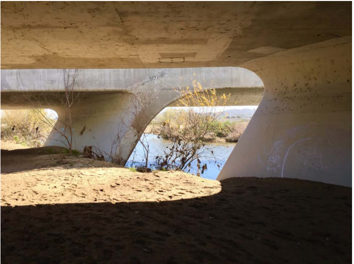
Burbank Boulevard overpass, upstream from the Sepulveda Dam. Image courtesy of Tyler Huxtable.
