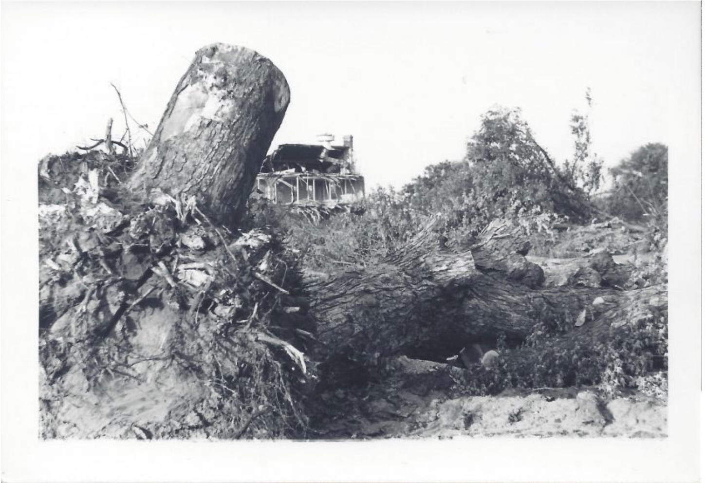
Barracks demolished for airport construction. Image by Richard E. Watson, M.D., courtesy of the author.
