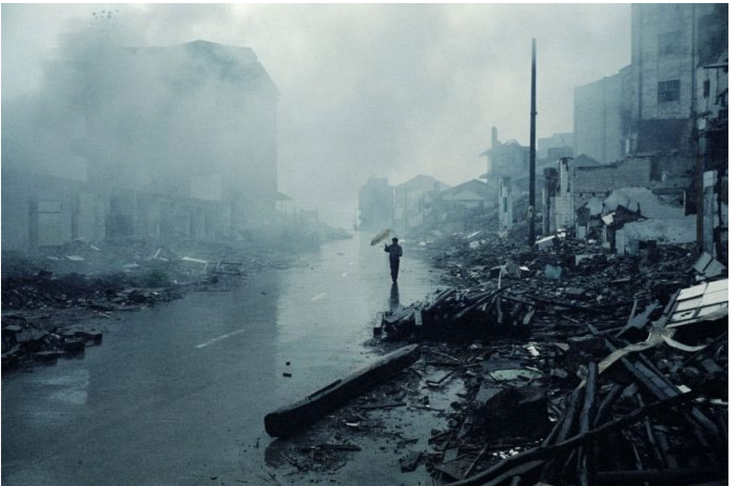
The destroyed old city of Wanzhou, only a few remaining local inhabitants are left behind. Mostly migrant workers remain to dismantle the city by hand and occasionally by using explosives. Wanzhou, China. 2002.
