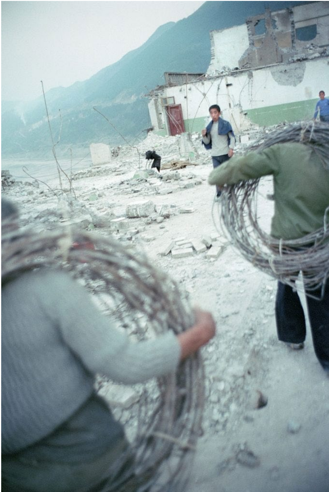
Migrant workers dismantling a recently vacated building. The workers supplement their poor income by selling scrap metal and bricks salvaged from demolition sites. Badong, China. 2002.
