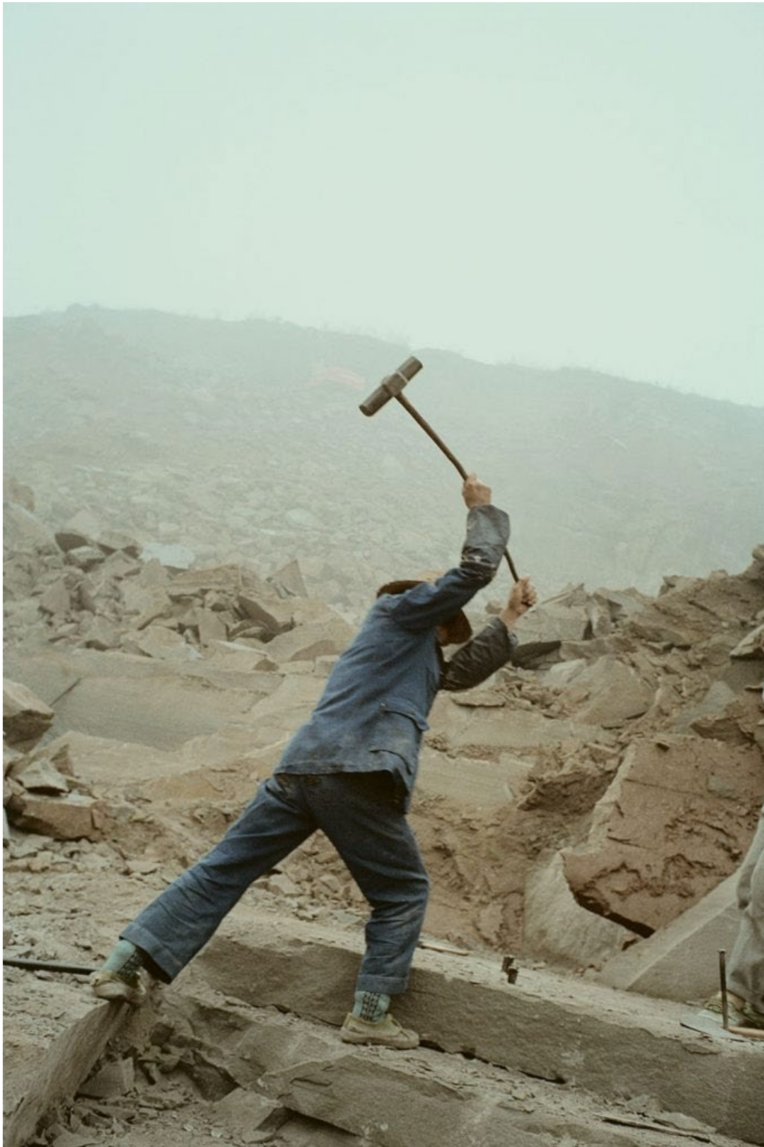
Migrant worker at a construction site in the new town. The town is built higher up the mountains and will replace the old town that will eventually be submerged upon the completion of the Three Gorges Dam. Yunyang, China. 2000.
