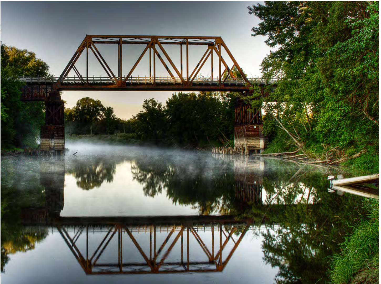
Steel truss bridge over the Mississippi River in Palisade, MN. Image courtesy of Peter Ladd, 2009.
