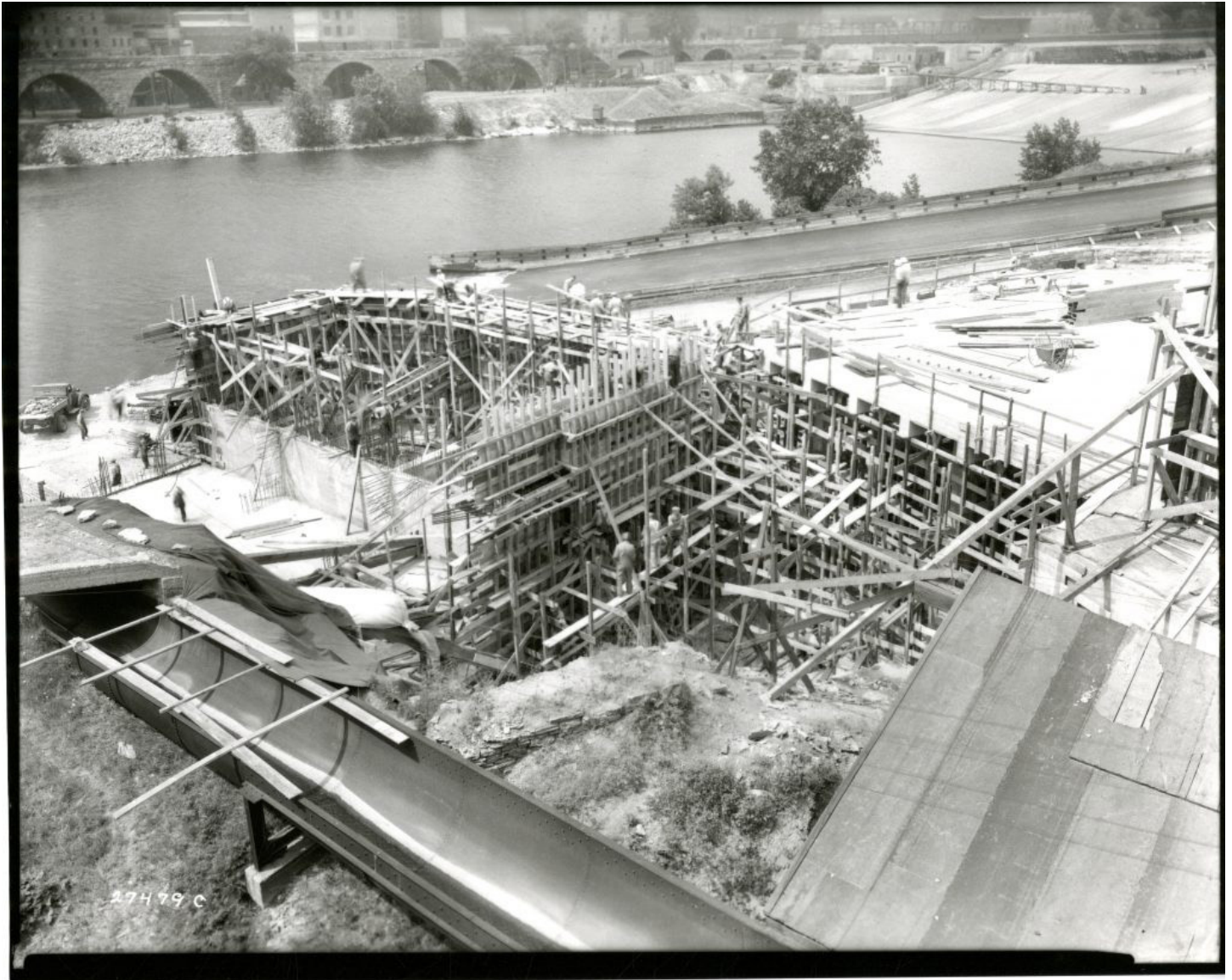
Construction of SAFL's volumetric tanks used for deep water research, the basement level used for experiments, and lower deck. The basement level was designed to flood when the river levels rose above a certain level. Notice the Stone Arch Bridge and St. Anthony Falls in the background.
