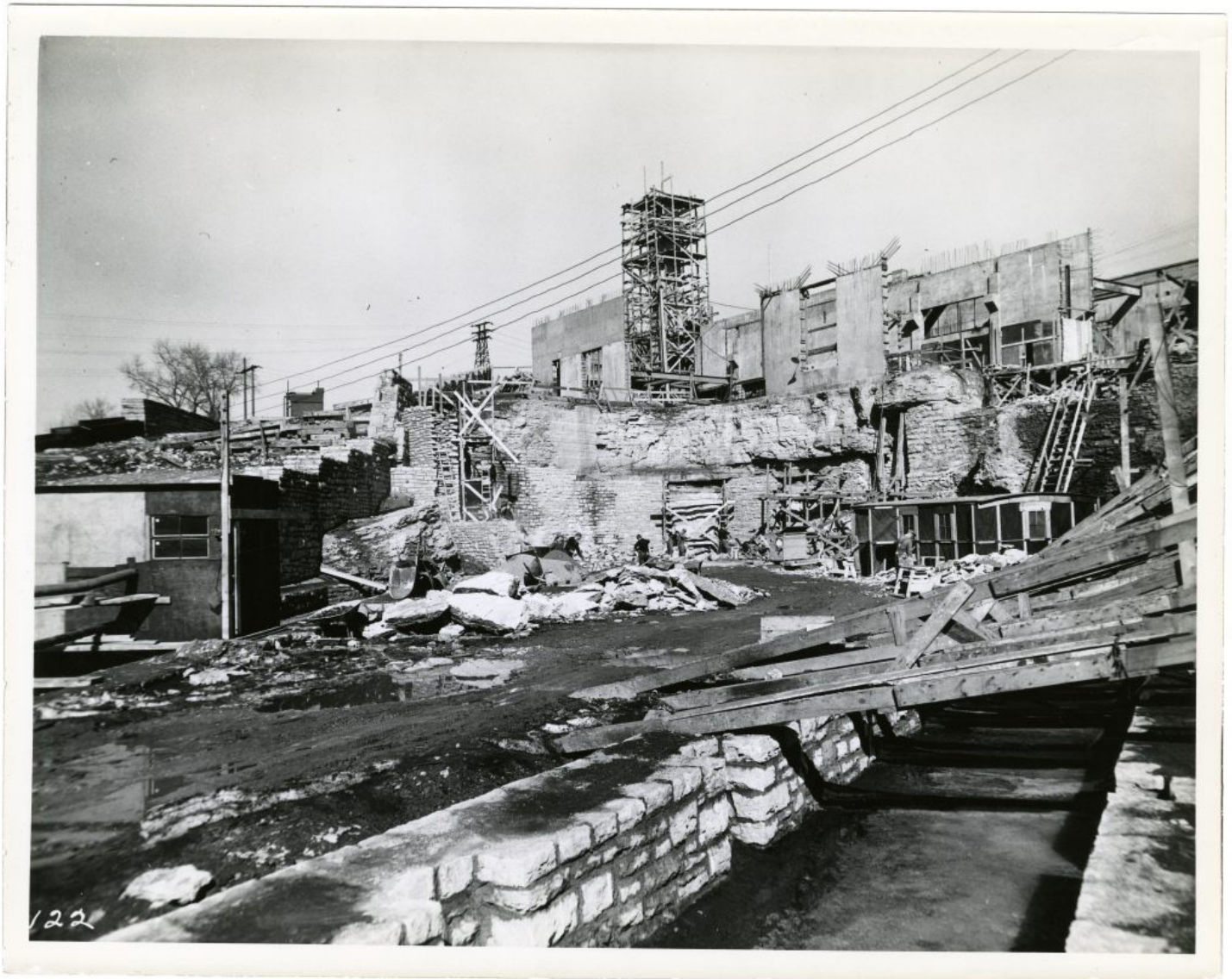
Laboratory construction in 1936 included excavation of approximately 30,000 lbs of limestone to expand the bottom floor where SAFL's outflow channel takes diverted water back to the river below St. Anthony Falls.
