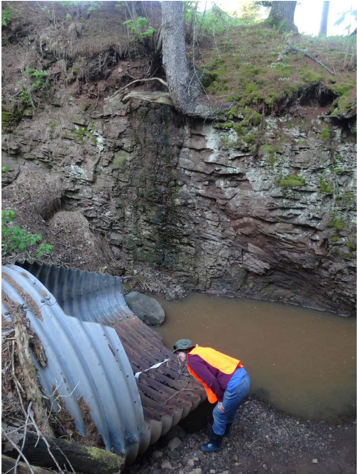
NRRI Field Technician Mary Heise inspects a large culvert in rural Duluth, Minn., as part of an effort to develop ditch and culvert best practices leading to protecting water quality. Image courtesy of Andrea Crouse.
