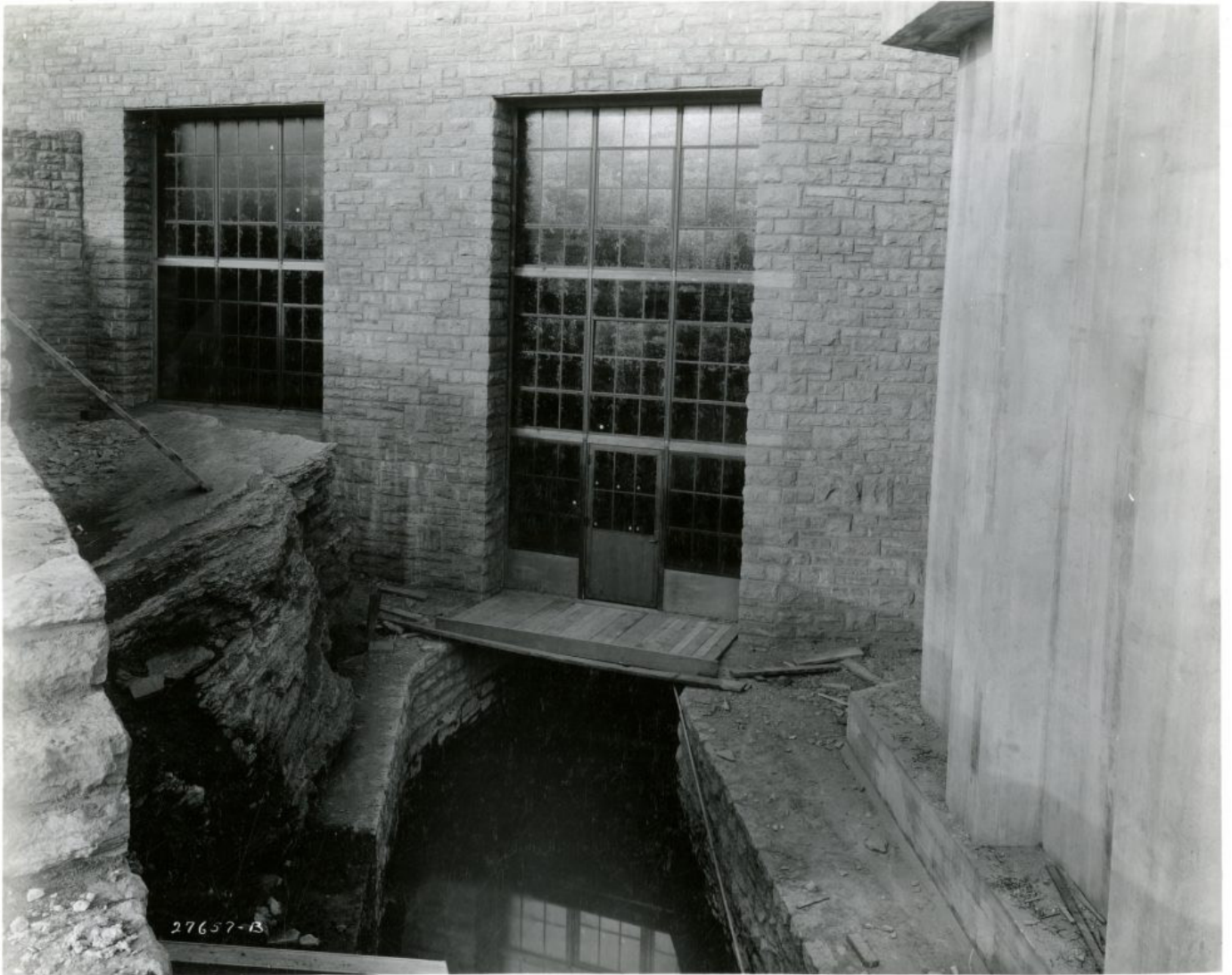
The basement level of the laboratory is constructed over the top of the outflow channel where water exits the building and rejoins the Mississippi River below the falls.
