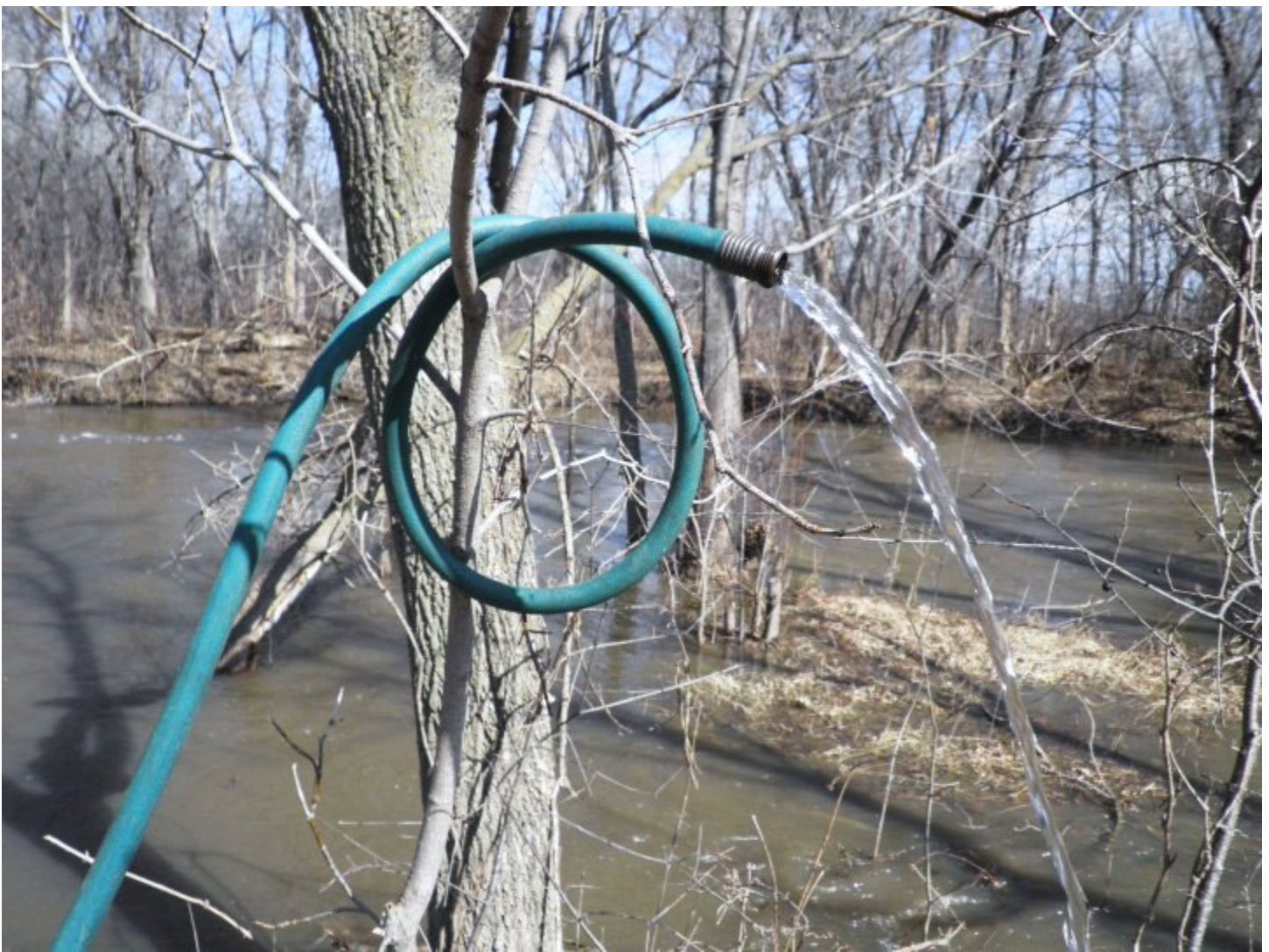
The sump pump that was pumping water out of my basement during the spring 2010 flooding. Firefly Creek, shown in the background, had risen approximately seven feet from the usual water level. I recall our household having to leave the sump pump going 24-7 for about two weeks. Image courtesy of Tianna M. Odegard.
