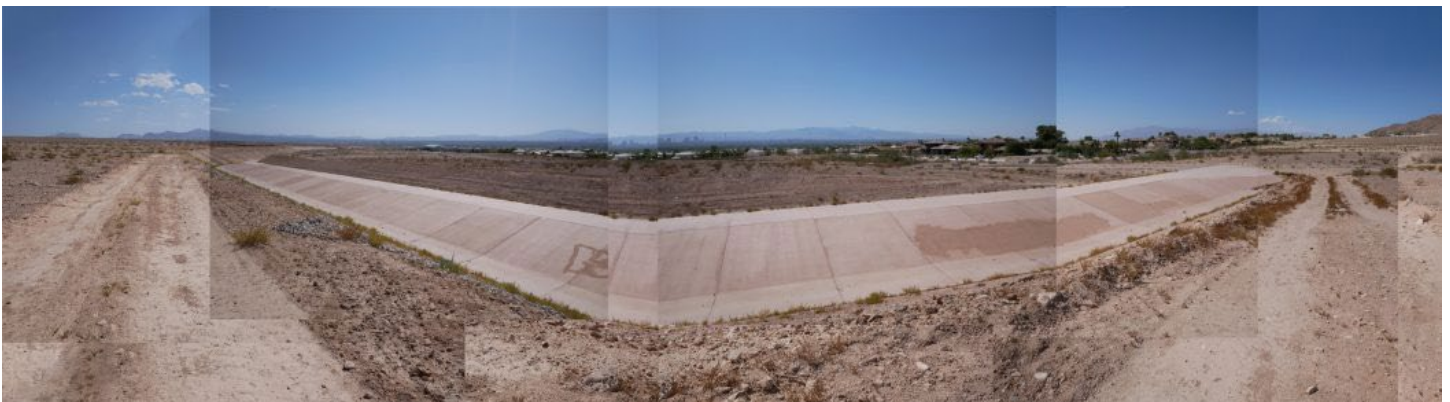
Water infrastructure at the eastern edge of Las Vegas that intercepts flood water coming off of Frenchman Mountain. Image courtesy of the author.
