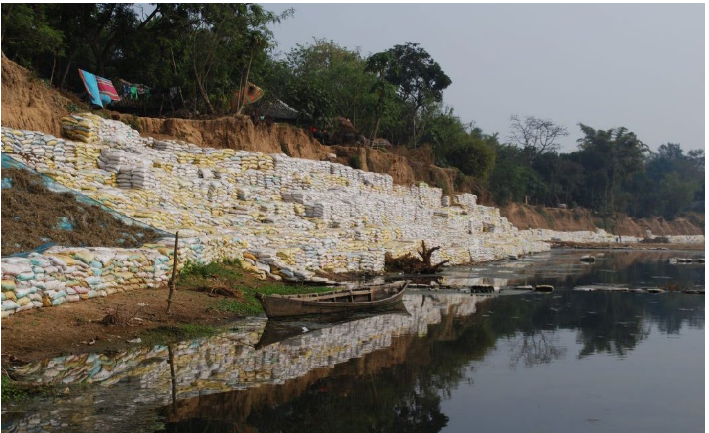
A temporary embankment near Dakshin Damurkholra. Image courtesy of the author.
