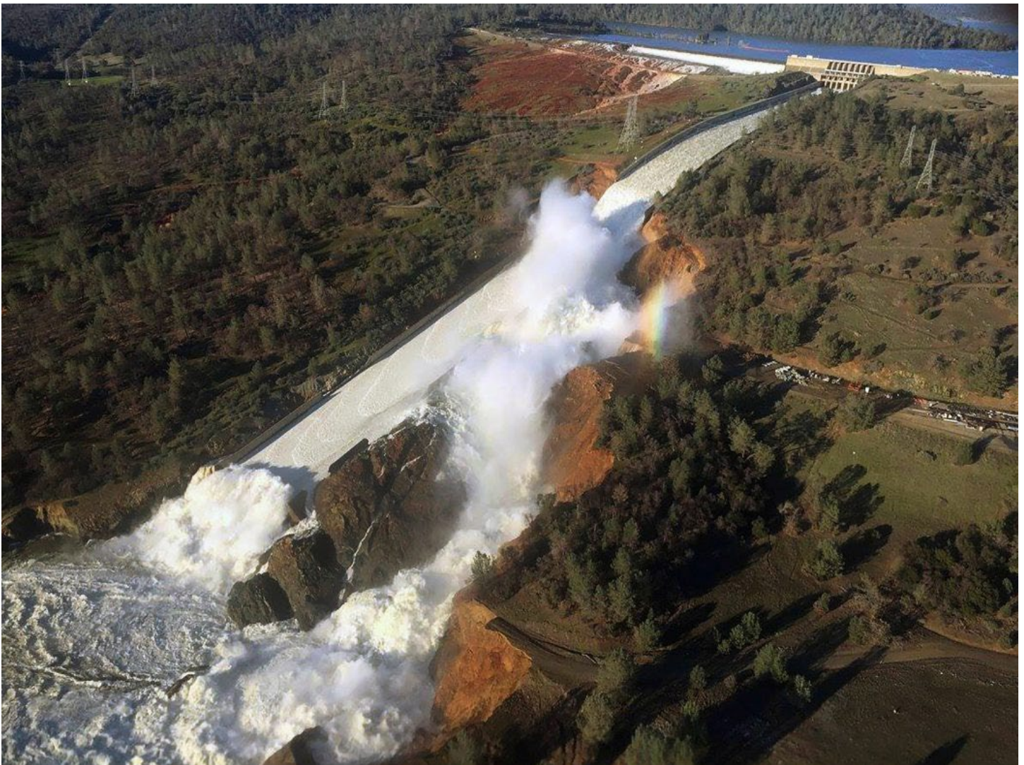
This aerial photo, released by the California Department of Water Resources, shows the damaged spillway with eroded hillside in Oroville, California during the dam crisis in 2017 during which the dam threatened collapse. This crisis remains emblematic of greater issues of water security globally and in California. Image by William Croyle, California Department of Water Resources.
